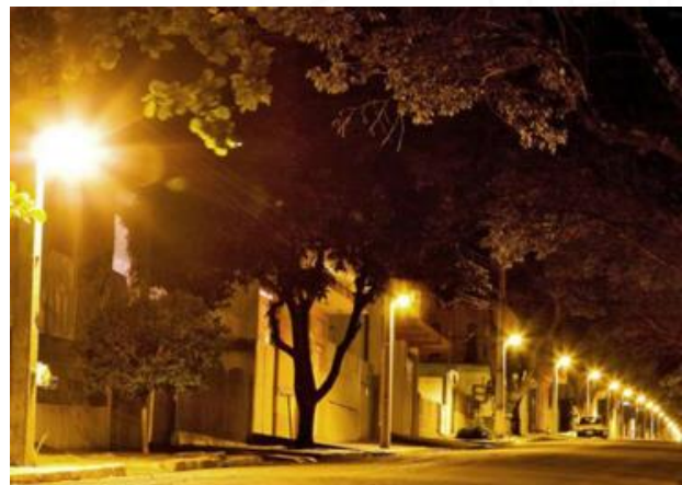
"Pilot of LED technology around the Cathedral of Maringá
